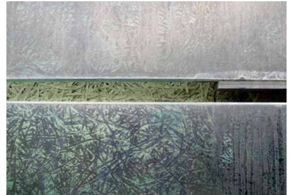
Figura 6. Herzog & De Meuron, Pfaffenholz Sports Centre, St. Louis, 1989-1993. The outer glass sheets of the envelope, with their silkscreen texture, imply transparency and appear to reveal what lies beyond, but they actually only allow the constitutive layers of the cladding to be seen, i.e. the compressed chipboard Eraclit panels, installed below. Here too the cladding purpose of the outer skin becomes explicit, despite the difficulty for viewers to fully perceive its depth.
