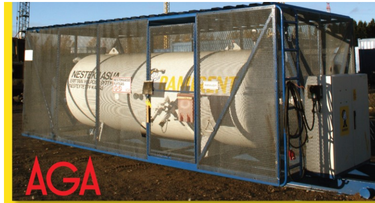
Figure 19 Liquid gas container on construction site (Aga 2017)
