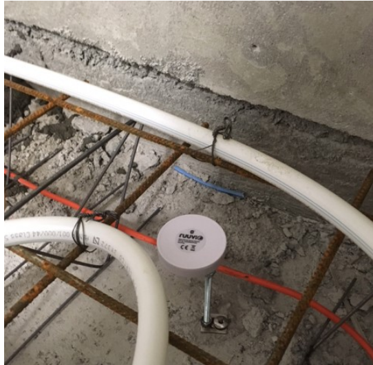
Figure 58 The RuuviTag was adjusted to 115mm, the orange curing cable can be seen
