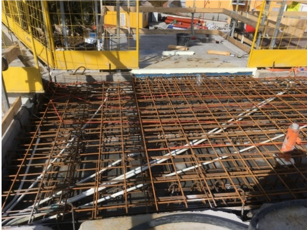
Figure 9 Significant amount of steel reinforcement is needed to fulfill the strength requirements of Schöck - balcony joints in the case study project
