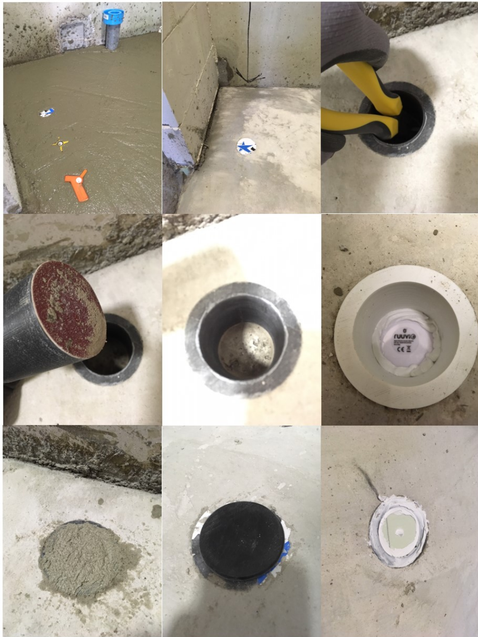
Figure 60 The installation process of RuuviTag sensors. In the upper left picture also the two Wiiste sensors can be seen in the concrete.
