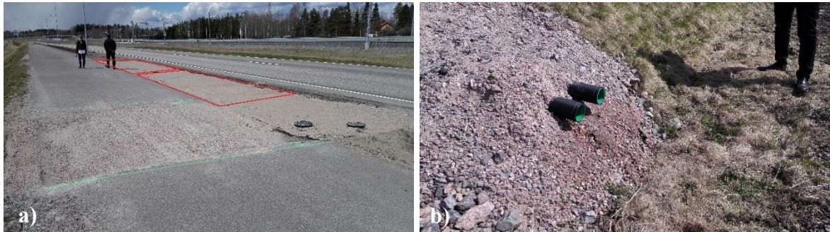
Figure 6. a) Upper parts of the sand filter (left) and sand-biochar filter (right) highlighted. The manholes in front connect the subsurface drains and outlet pipes which convey water under the walkway to the left. Gravel part of the walkway was covered with new asphalt before the beginning of the study. b) Drain outlets from the sand filter (left) and sand-biochar filter (right) discharging into the ditch next to the road.
