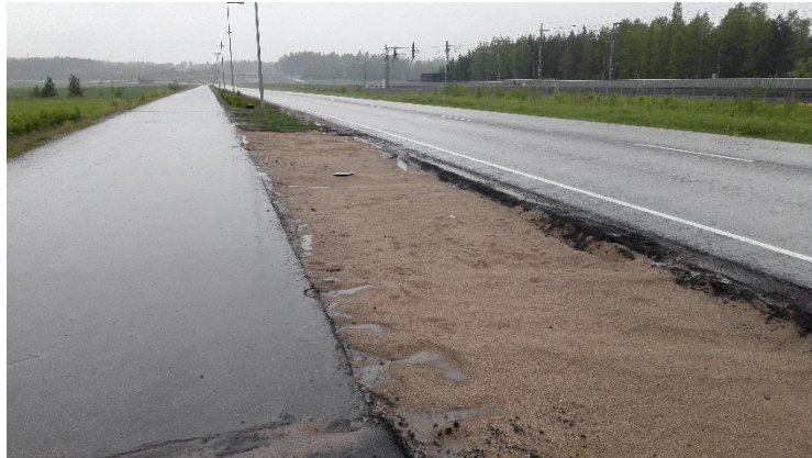
Figure 17. The filters during the rain event in June 8 (19:14). Temporary ponding was observed on top of the filters due to intensive rainfall.
