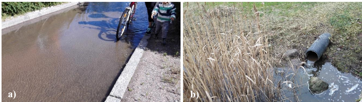
Figure 1. Small-scale quantity (a) and quality (b) problems related to stormwater. a) Stormwater flooding on a walkway long after rainfall. b) A stormwater sewer discharging into an urban stream habituated by endangered sea trout.
