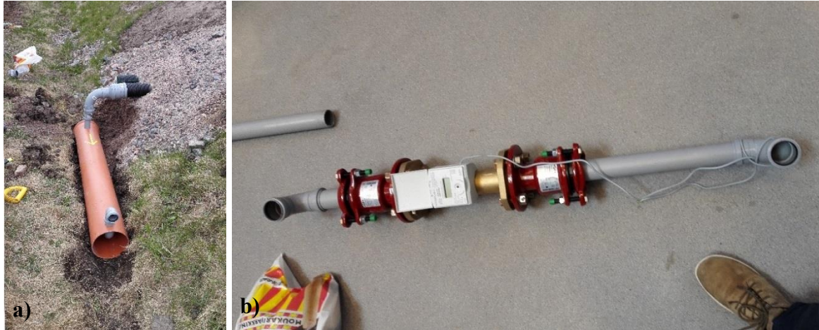
Figure 12. Installation of the automatic effluent flow rate meter for the sand-biochar filter. The flow rate meter, its transmitter (not shown) and pipes (grey) are placed inside the bigger red pipe, which protects the devices. Water samples and manual flow rate measurements were taken from the outlet. Note that the outlet is higher than the water meter to ensure it is constantly full of water.
