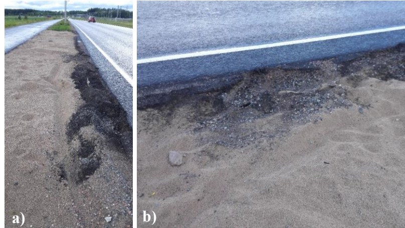
Figure 19. Vehicle had driven over the filters and damaged the structure revealing the edge of the filter fabric or bentonite mat. Some of the stormwater from the road surface may have infiltrated to the ground outside the filter.
