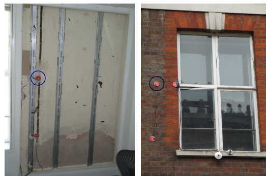
Figure 3. Internal (left) and external (right) view of the solid brick wall (SWall) case study. Circled in blue are the pair of sensors analysed.
