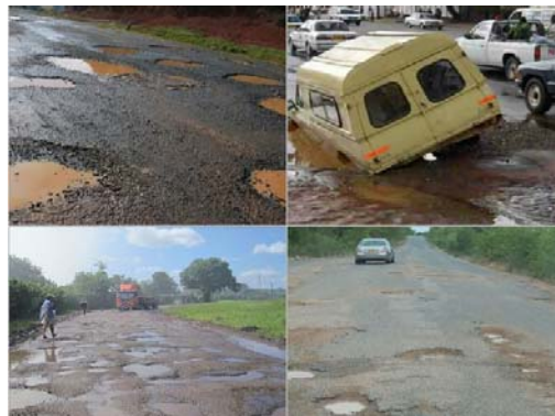
Figure 1. State of Zimbabwe's Roads in 2017.
