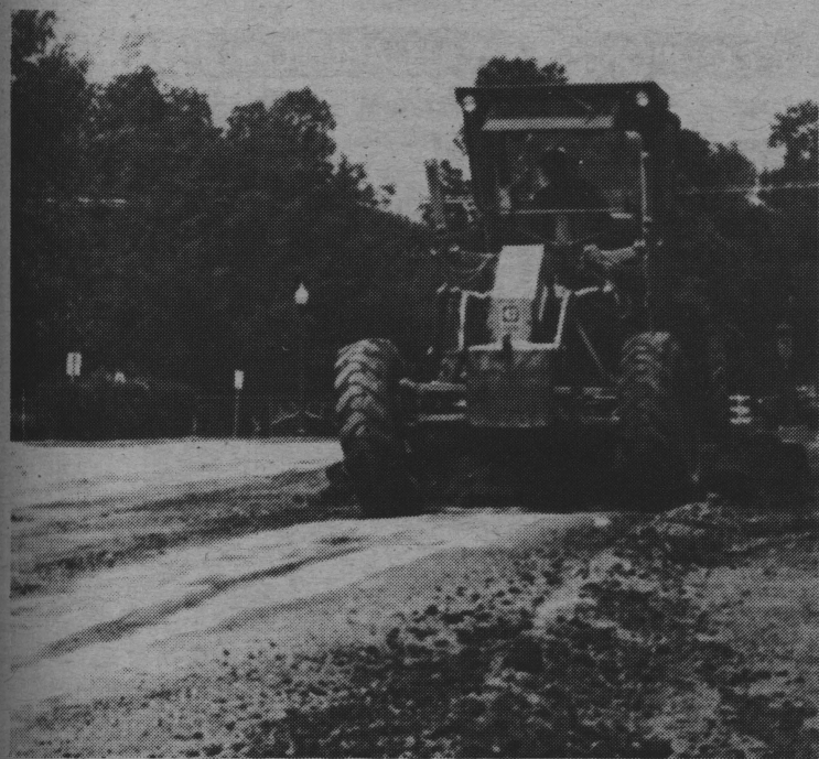
The only vehicle that has been able to drive down Ninth Street lately has been this earth excavator. (News photo by Mike Prizy)
