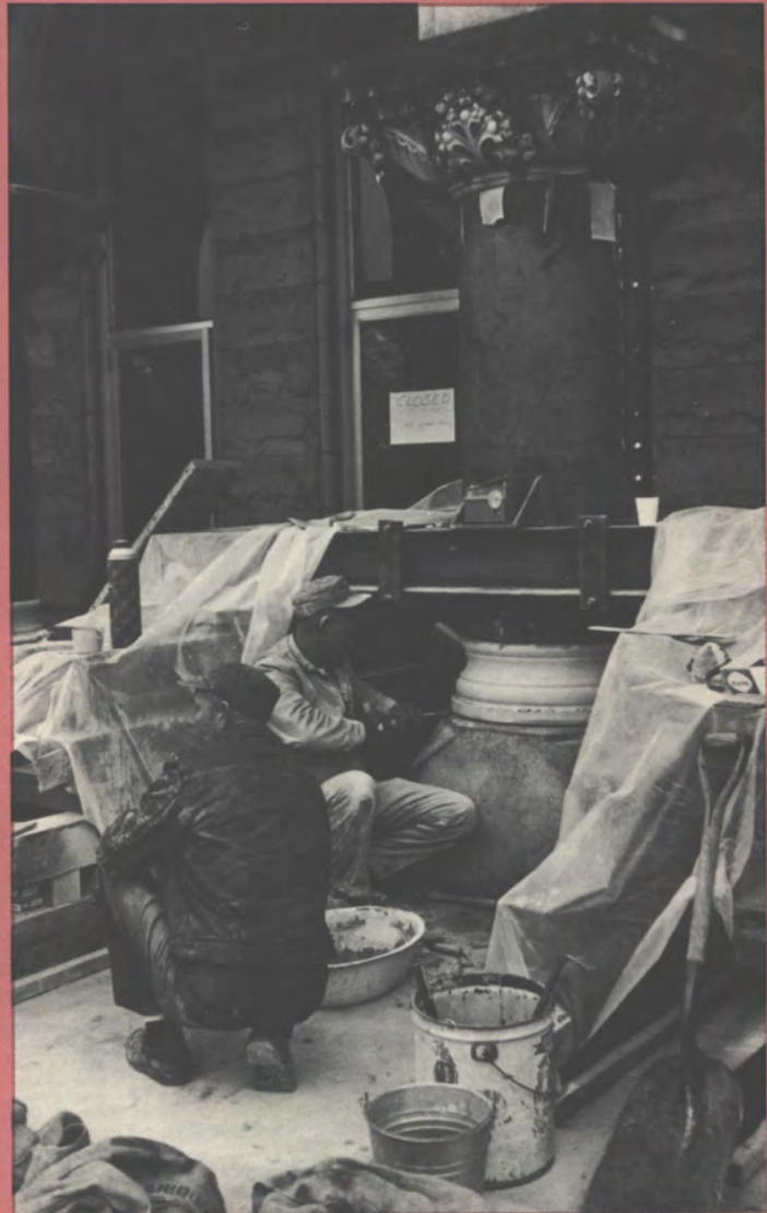
A sizeable amount of the biennium's budget goes for repairs of present edifices. The marble columns of Old Main were hypersensitively renovated in November of 1967 when new stone bases were added and the old, cracked ones removed.
