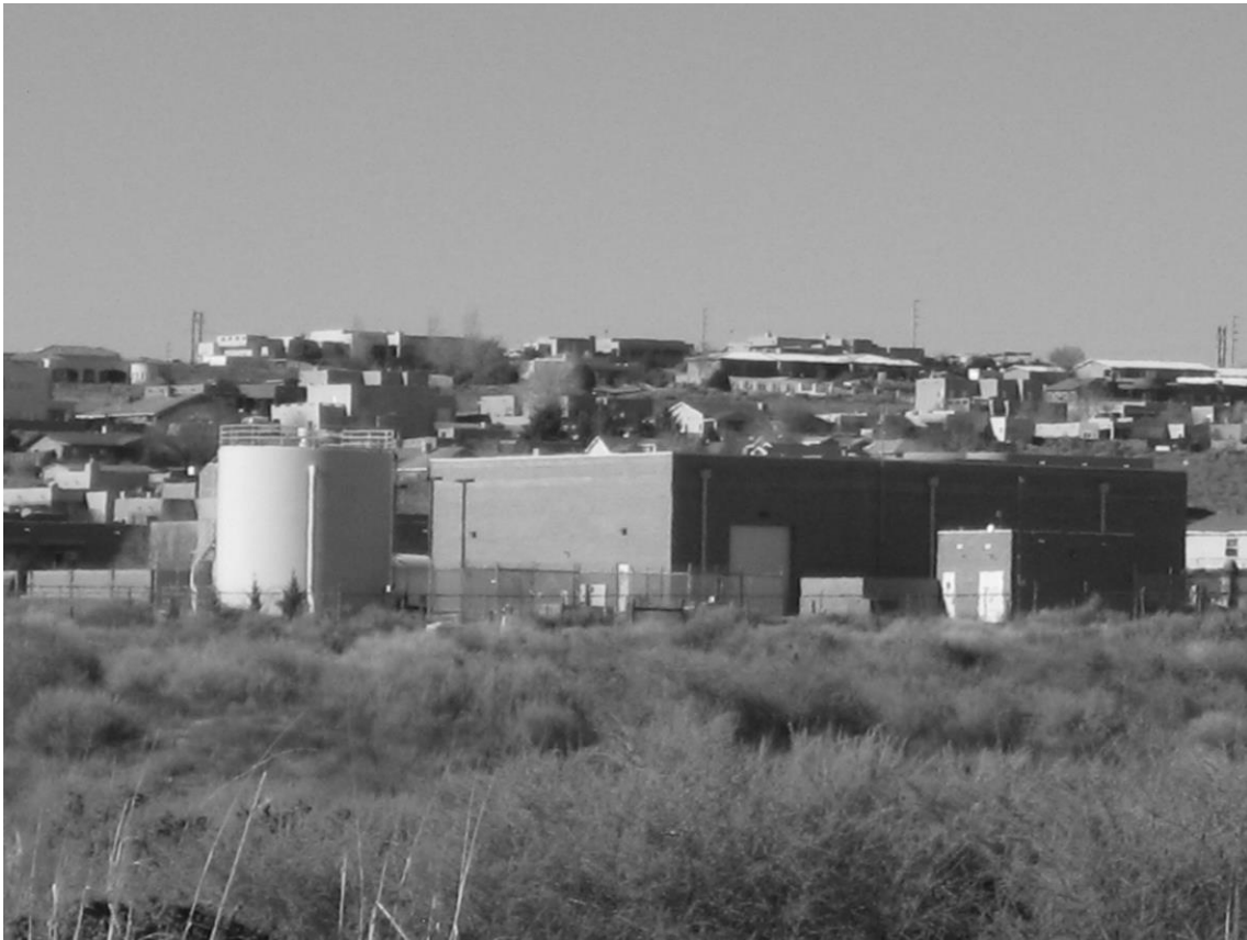
Figure 3. Ground view of reservoir tank and building housing one of the 17 wells currently used as water supply to Rio Rancho.
