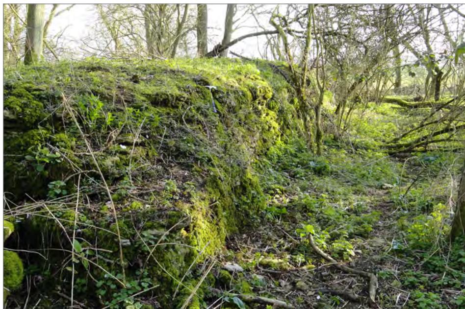
(b): Torpel Lodge remains: northwest corner, looking south externally. The coursed rubble walling would have been originally faced with limestone ashlar. The corner in the foreground appears to have carried pilaster buttresses.
