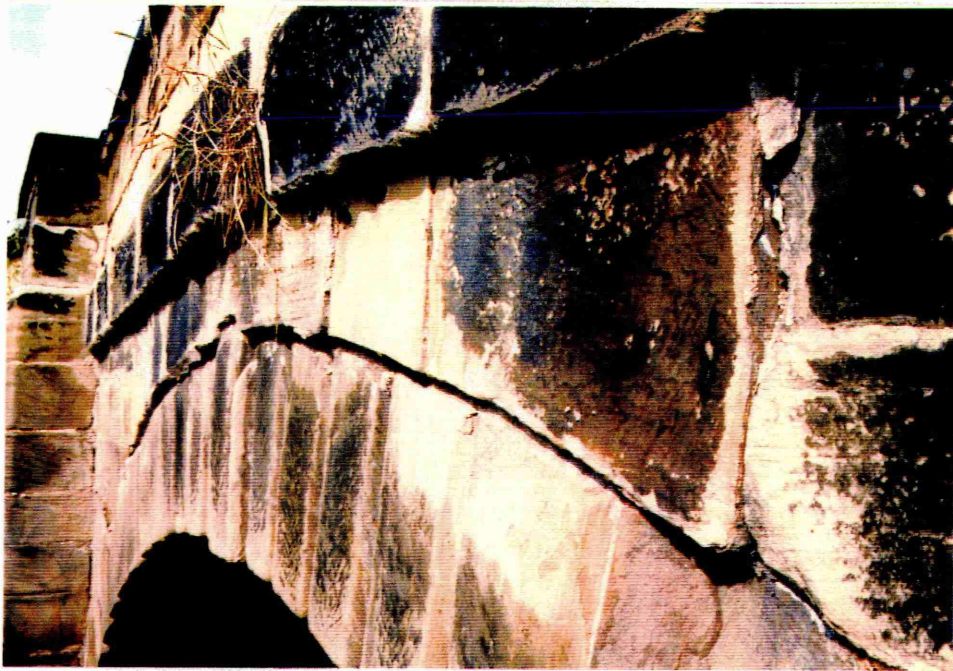
Plate 2.9 Bolton Mill Bridge, South Yorkshire, Showing Overall Poor Condition.
