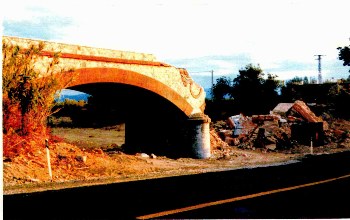
Plate 2.12 Note Increase In Parapet/Spandrel Wall Thickness (Background, Right) In This Same Example Of French Practice.
