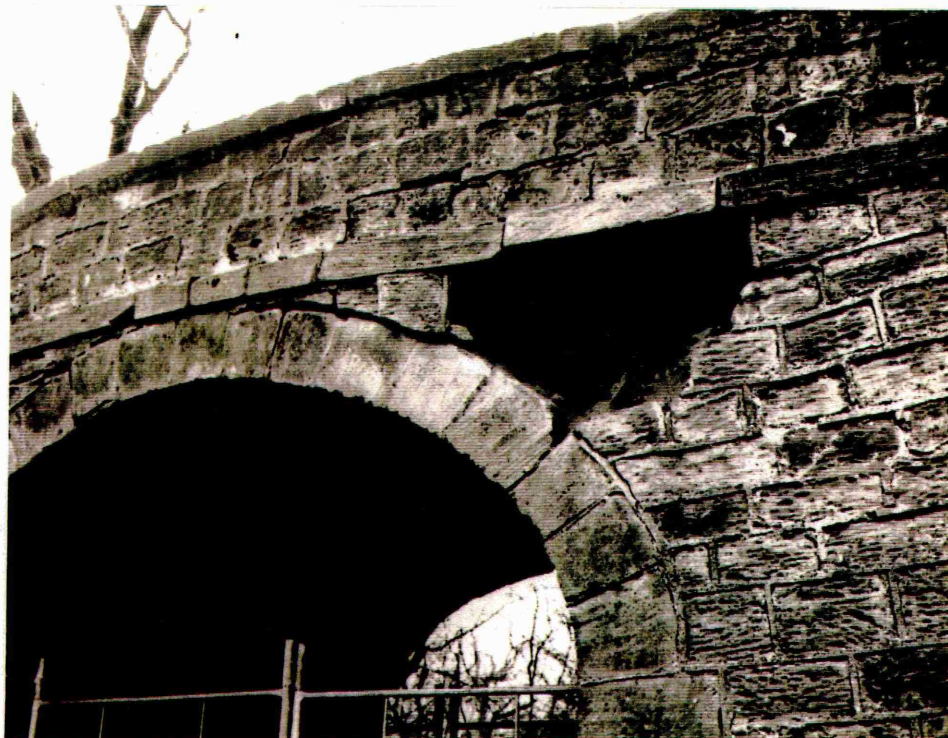
Plate 2.2 Burying Lane Bridge, After Passage Of Mining Wave, As At November 1975
