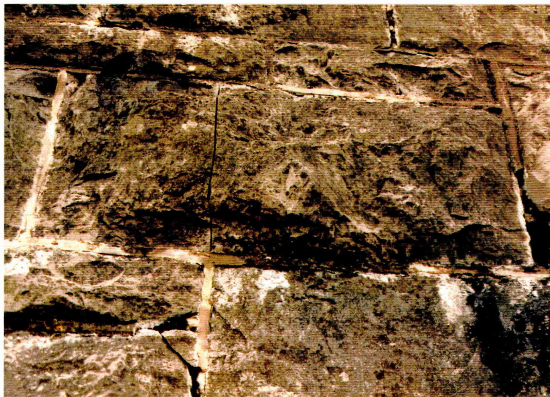
Plate 2.8 Typical Cracking On Ribbleshead's Masonry Piers
