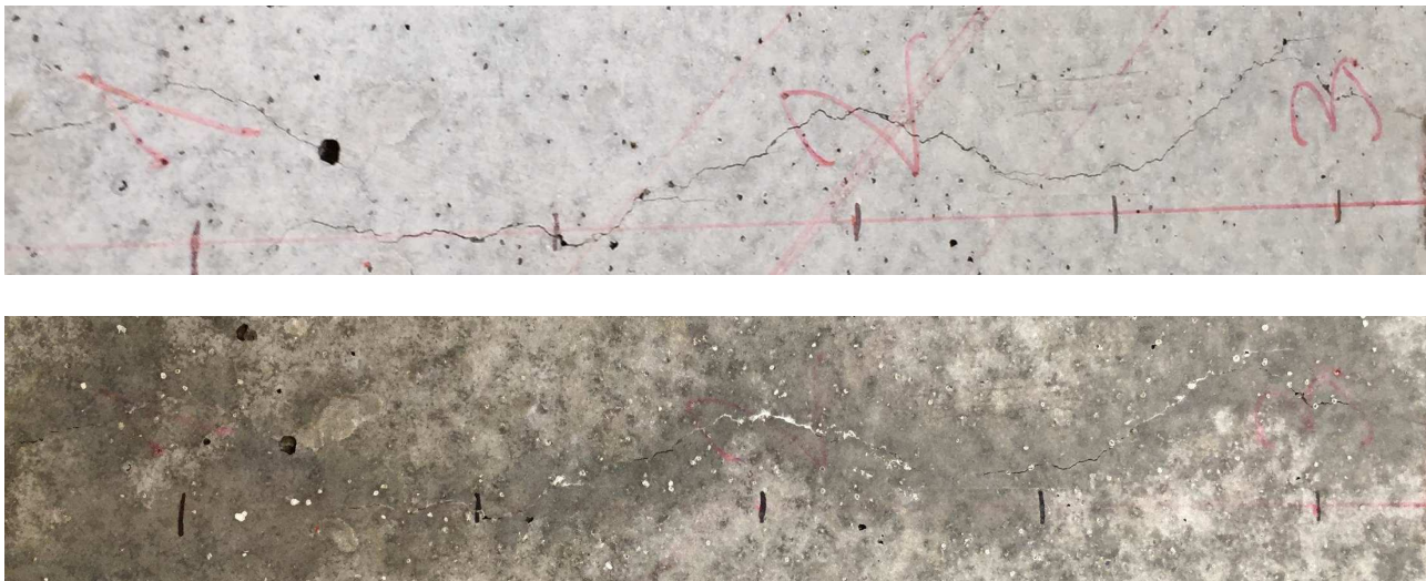
Figure 7. C-SAP beam with a 0.2 mm crack before (top) and after (bottom) 4 weeks water exposure.
