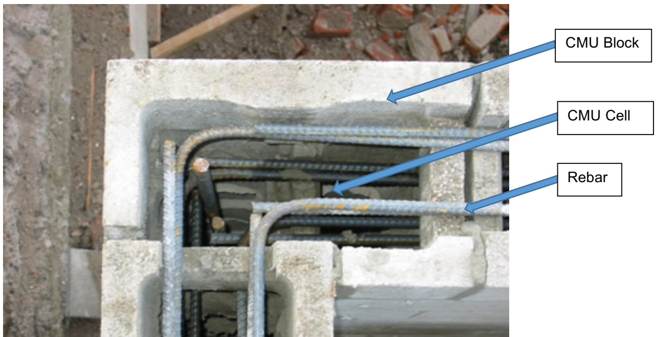
Figure 1: Rebar Congestion in CMU cell
