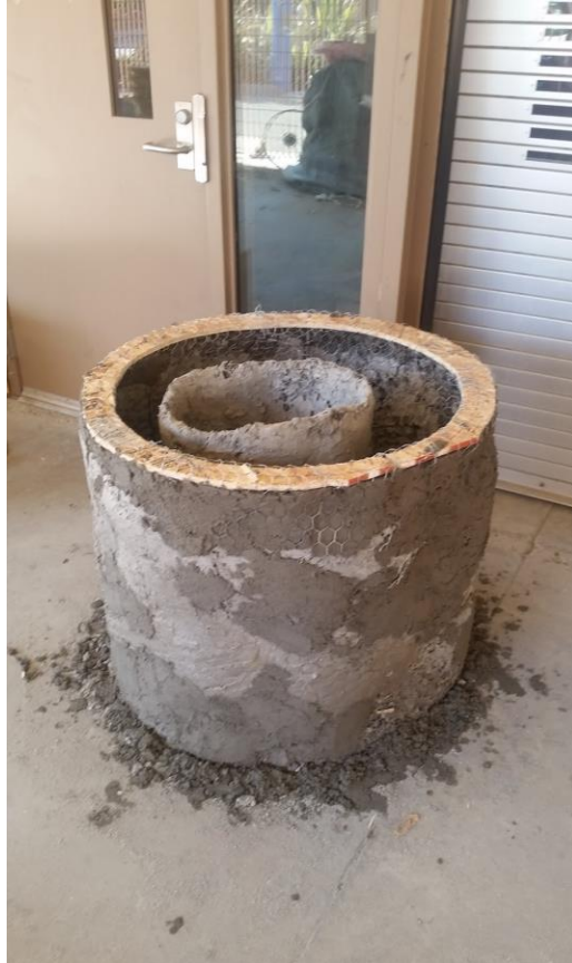
Figure 33. Outer walls of the thermal reservoir coated with stucco. This unit is nearly complete. A final layer of stucco will be added over the plywood and to patch any gaps before it is finished.
