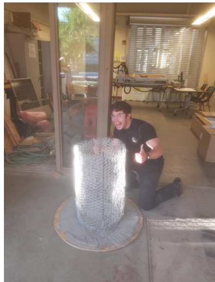
Figure 27. Spencer poses with the mesh and rebar backbone of the inner housing ring. Stucco has been applied to the plywood base to prevent the possibility of fire.
