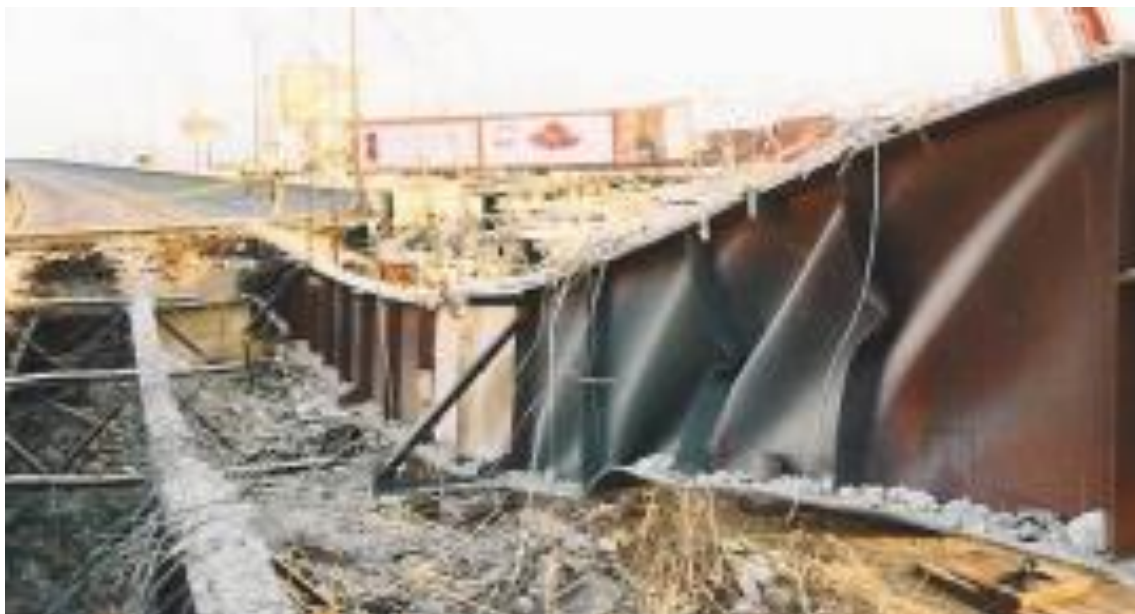
Figure 1.3 – Shear buckling in a steel plate girder after fire (Franssen & Vila Real, 2010)
