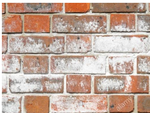
Figure 3. Salt crystallisation on brick wall
