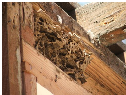
Figure 2. Termite damage on building structure
