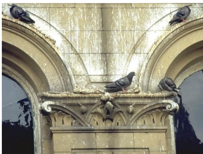
Figure 1. Bird damage on historical building
