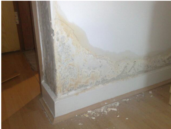
Figure 5. Rising damp on masonry wall
