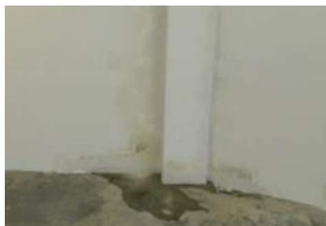
Figure 0. Imprint of water caused from rising damp
