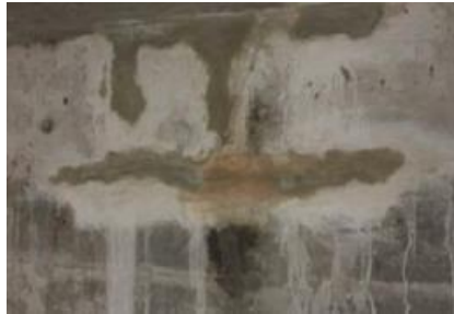
Figure 10. Leaking that can be found on the swimming pool wall
