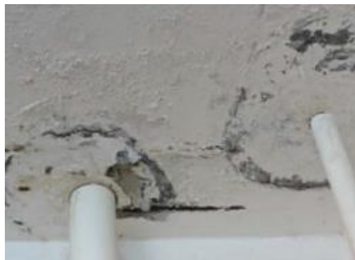
Figure 11. Cracking on the edge of planter box and deterioration of waterproofing on slab surface
