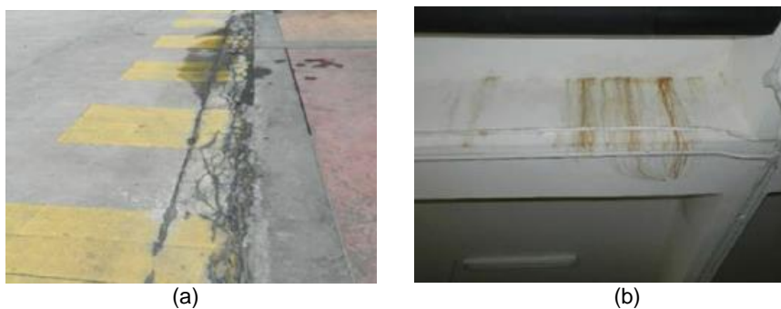
Figure 7. (a) Expansion Joint on the Parking lot surface and (b) the effect on structure below
