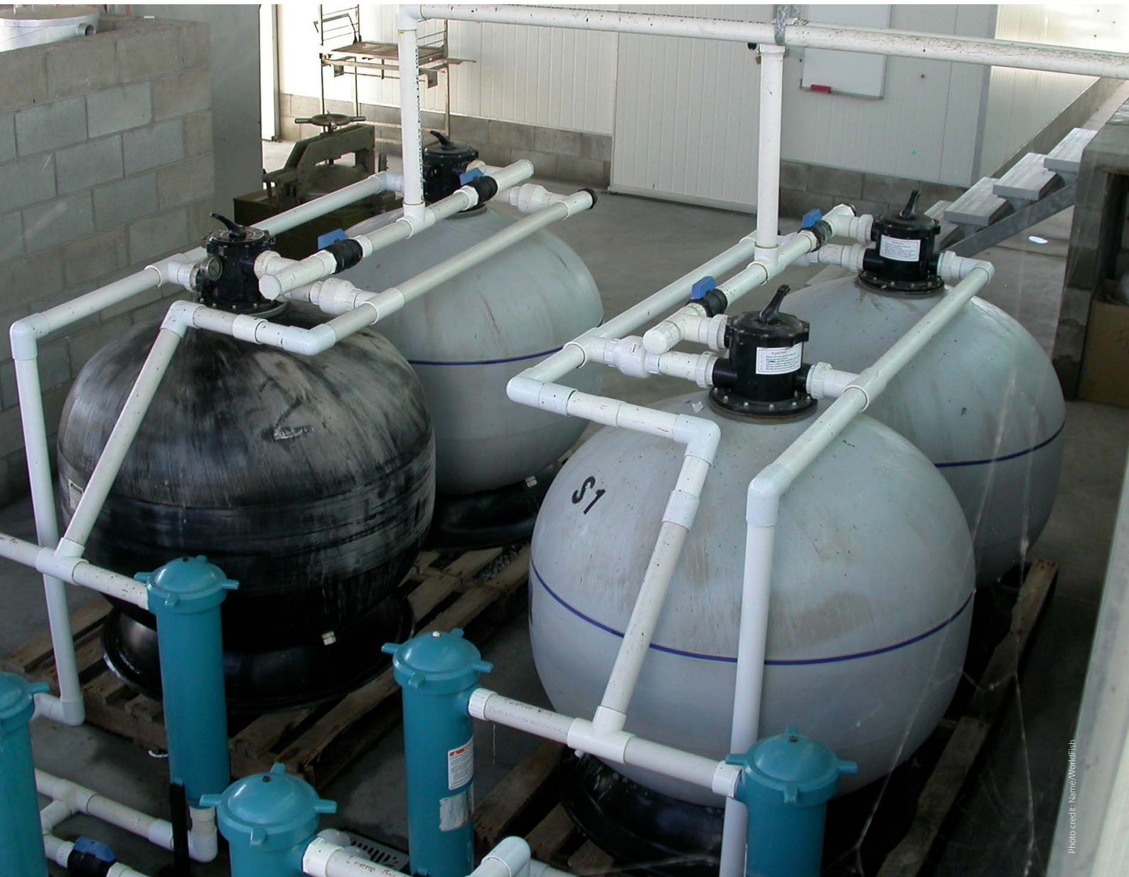
Sand filters and UV light used for treating the water supply to the hatchery.
