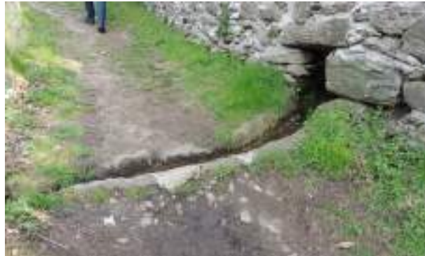
Fig. 4 - Ancient canalisation help the draining system of the drystone wall. (photo: Andrea L'Erario)
