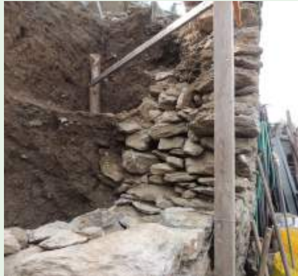
Fig. 28 - Section of a wall under construction: here the horizontal lay out of stones are clearly visible, the vertical alignment helped by a wood post, the difference between the big stones in the front and the small stones for the drainage at the back. (photo: Andrea L'Erario)
