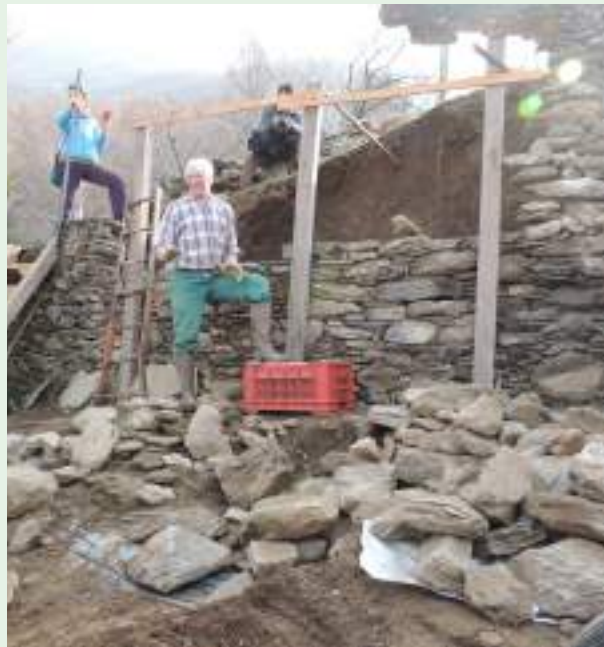
Fig. 31 - Accomplishing the repair of a wall provides great satisfaction! It is proud work! (photo Andrea L'Erario)
