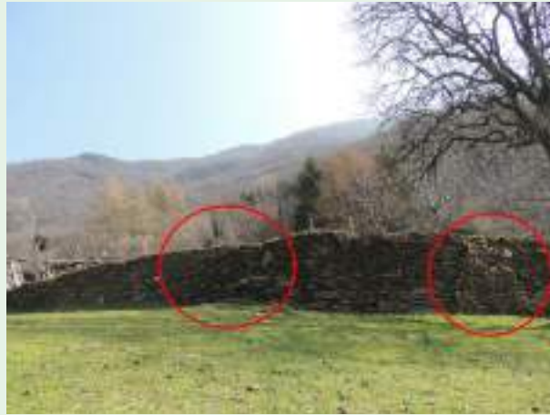
Fig. 30 - Two level junctions in the wall are visible in the red circle. (photo: Andrea L'Erario)
