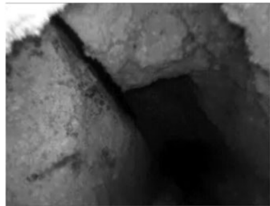
FIGURE 20 The cavity observed inside the pillar
