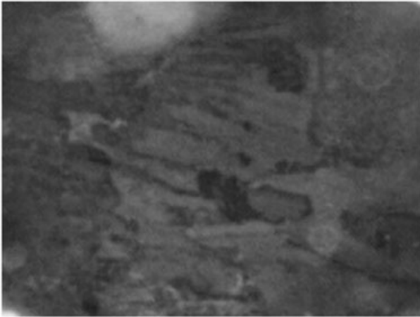
FIGURE 21 The wooden surface observed inside the pillar
