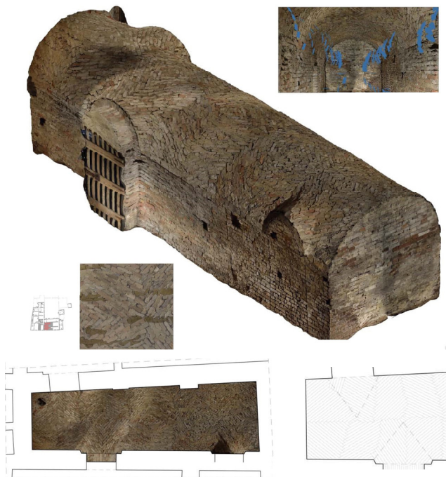
Figure 1. Magio Grasselli palace in Cremona: groined vaults in which the bricks were laid perpendicularly to the diagonal arches
