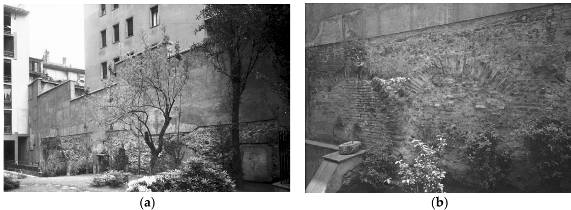
Figure 2. Photographs of the remains of the external wall of the circus visible in a private garden of a building in via Vigna 1: (a) the entire portion of the remains; (b) a detail of the arches sustaining the podium visible on the wall (courtesy of Ministero dei beni e delle attività culturali e del turismo).
