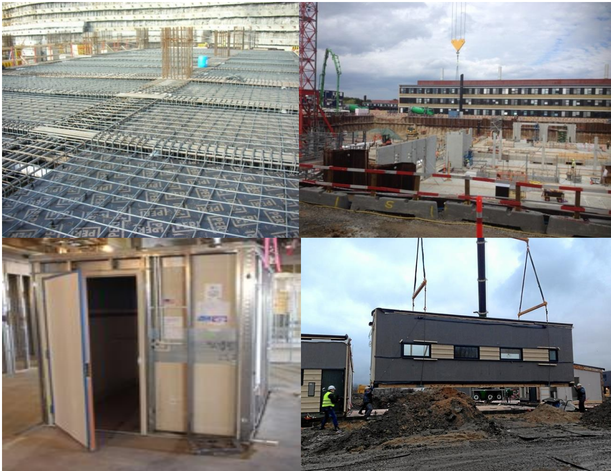
Figure 18. Top left: Component manufacture and sub-assembly Zorlu Center Project Istanbul, 2009; top right: Non-volumetric pre-assembly DTU Life Science Building 2014; bottom left: Volumetric pre-assembly, Mortenson Construction, Saint Joseph Hospital in Denver, Colorado, bathroom pod, from Modular Building Institute, and bottom right: Modular building, Scandi Byg from Licitationen 3 August 2016.
