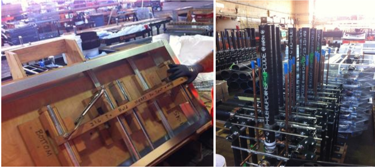
Figure 47. Welding jig used as frame on the left and stock of prefabricated modules on the right, 13 October 2015.
