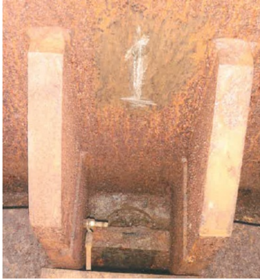
Figure 3: Photograph of the bracket inside the wind turbine, Fig. 1b. The bracket is subject to severe corrosion. Photograph from Ørsted ® .
