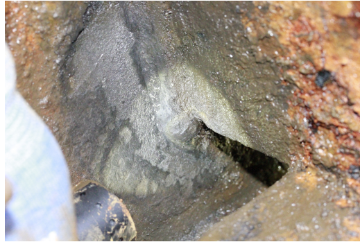
Figure 1: Welded component inside a wind turbine foundation under the Transitional Environmental Protection (TEP) process. The weld was protected against corrosion for a certain operational time. Afterwards, a leakage generated a corrosive environment. Photograph from Ørsted®.
