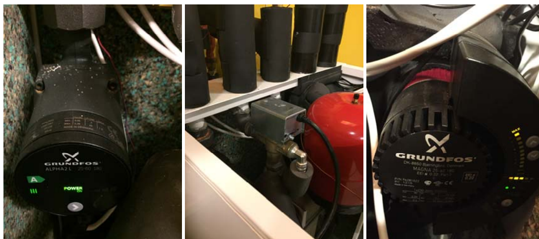
Figure 9. The two pumps and the 3-way motor valve in the heat pump.
