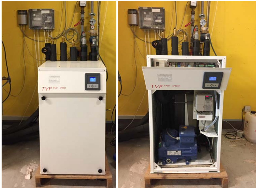
Figure 8. Pictures of the heat pump.
