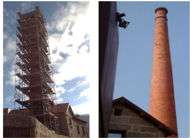
Figure 3. Structural intervention in the chimney: (a) view with the scaffolding for the works execution; (b) final configuration.
