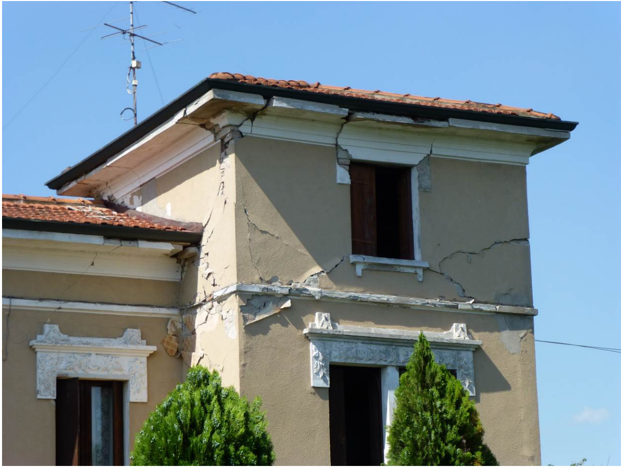
Fig. 9. Damage around an opening in a clay brick masonry building after the Emilia 2012 earthquakes (photo by L. Sorrentino).
