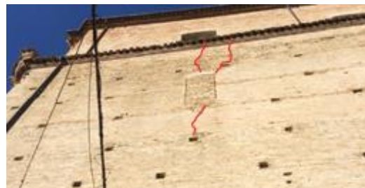
Figure 8: Church 3, Madonna della Misericordia in Petriolo. -a: façade photo. -b: internal view. -c: deep crack on the lateral wall, from inside. -d: crack pattern on the façade. -e: apse vertical crack. -f: crack on the lateral wall, from outside.
