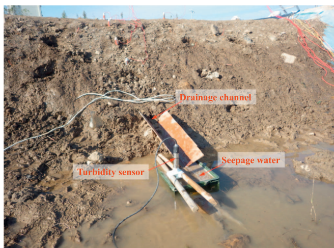
Fig. 7. Turbidity sensor to monitor the rate of internal erosion and piping.
