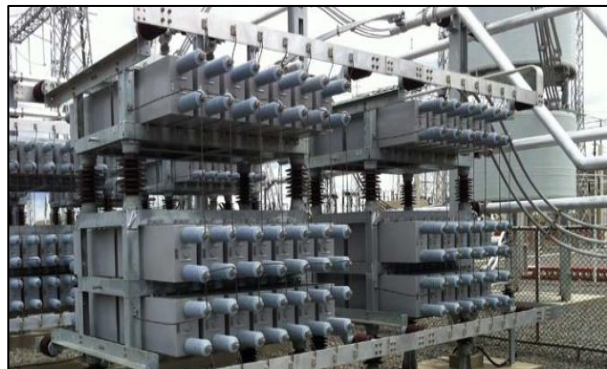
Figure 2.2- 6: SVC Sapeaçu Capacitor Bank [26]
