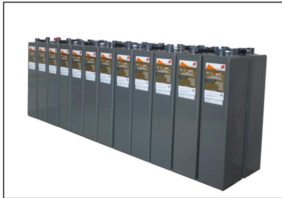
Figure 2.2- 4: Battery Bank Storage [25]
