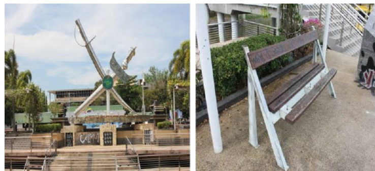
Figure 4. Poor condition of facilities, safety, vandalism and lack of maintenance along the waterfront
