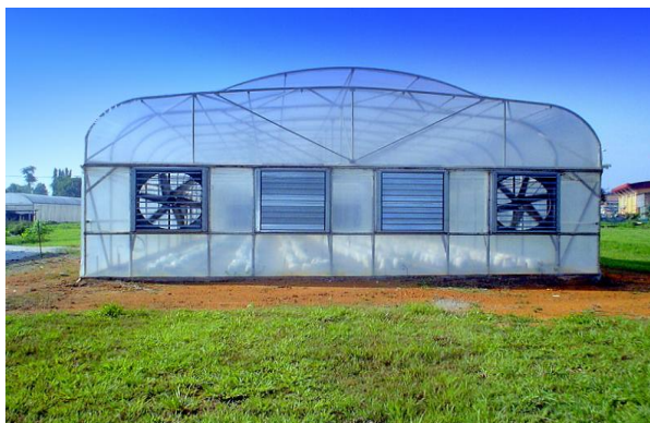
Fig.2: Exhaust fans placed at the north wall of the greenhouse
