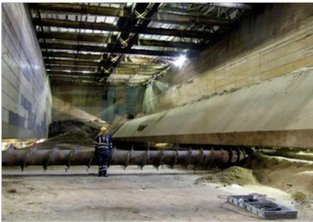
Figure 33 The Netherland 36.5MW biomass power plant using chicken manure to power 90,000 Homes. The plant will convert one third of the country's total 1.2 million tons of poultry waste produced per year.
