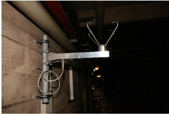
Figure 22: Ultrasonic anemometers install in the tunnel
