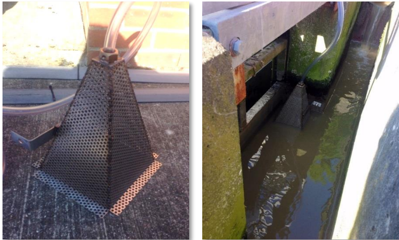
Figure 2.2 Photograph of stainless steel pyramid filter installed in the open channel at Fishburn STW. The filter, which had 6 mm apertures, was designed to prevent clogging in the pilot scale MEC.
