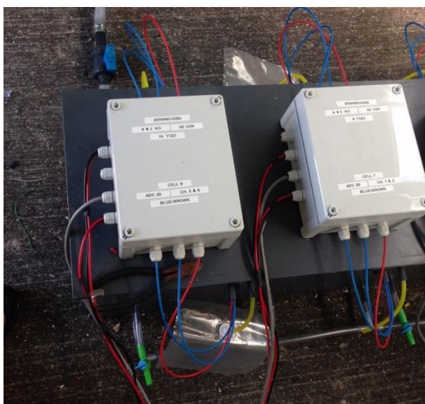
Figure 2.3. Photograph of MEC wiring and IP65 rated weatherproof boxes at Fishburn. Boxes were labelled with the corresponding module, data logger and channel for ease of identification. Liquid sampling ports can be seen protruding the tank (green and blue taps).
