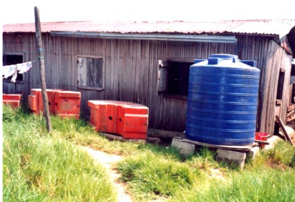
Figure 6.12: Rainwater Harvesting in NDR Source: Fieldwork, (2013).
