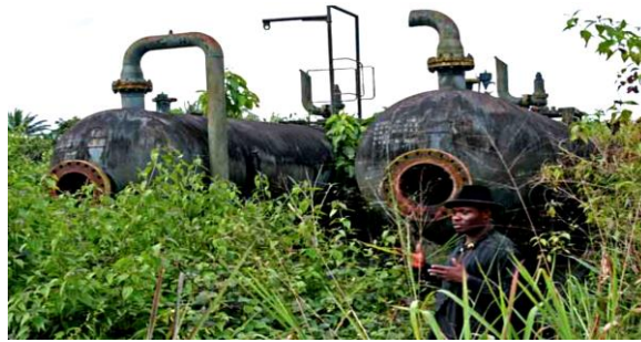
Figure 6.20: SPDC’s Oil Facility in decommissioned site overgrown with vegetation in NDR
