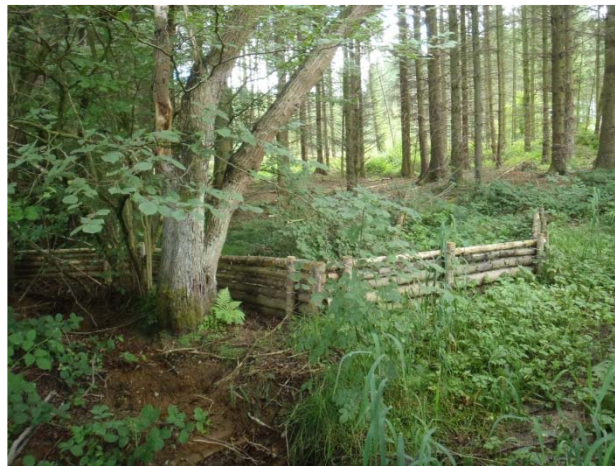
Figure 5-26 Looking upslope at a wooden barrier feature at site 4 for attenuating overland flows
