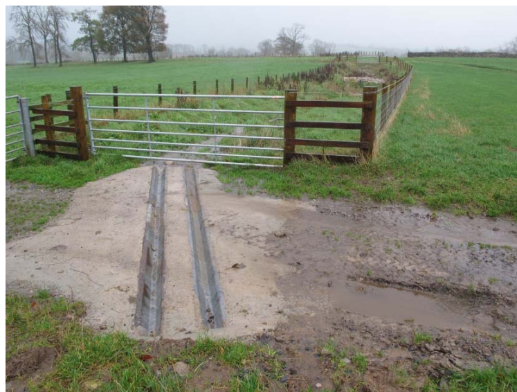
Figure 4-19 Photo of track runoff diversion in to a RAF
