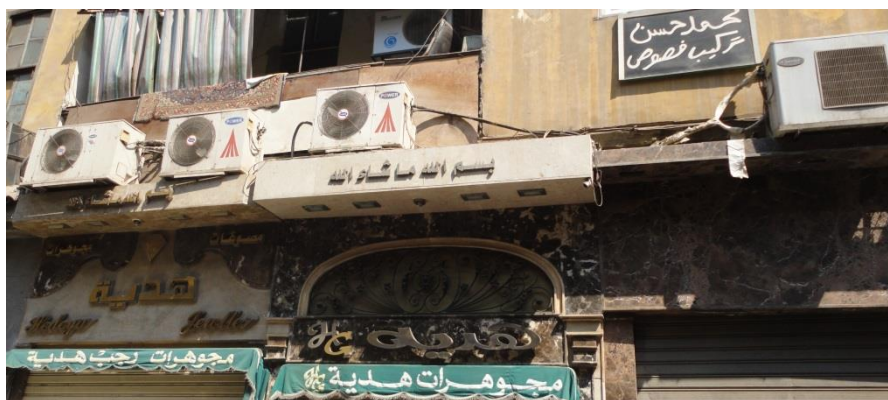
Figure 5-16 The excess heat is emitted from the mechanical ventilation to the urban air, which may increase the air temperature in the street
