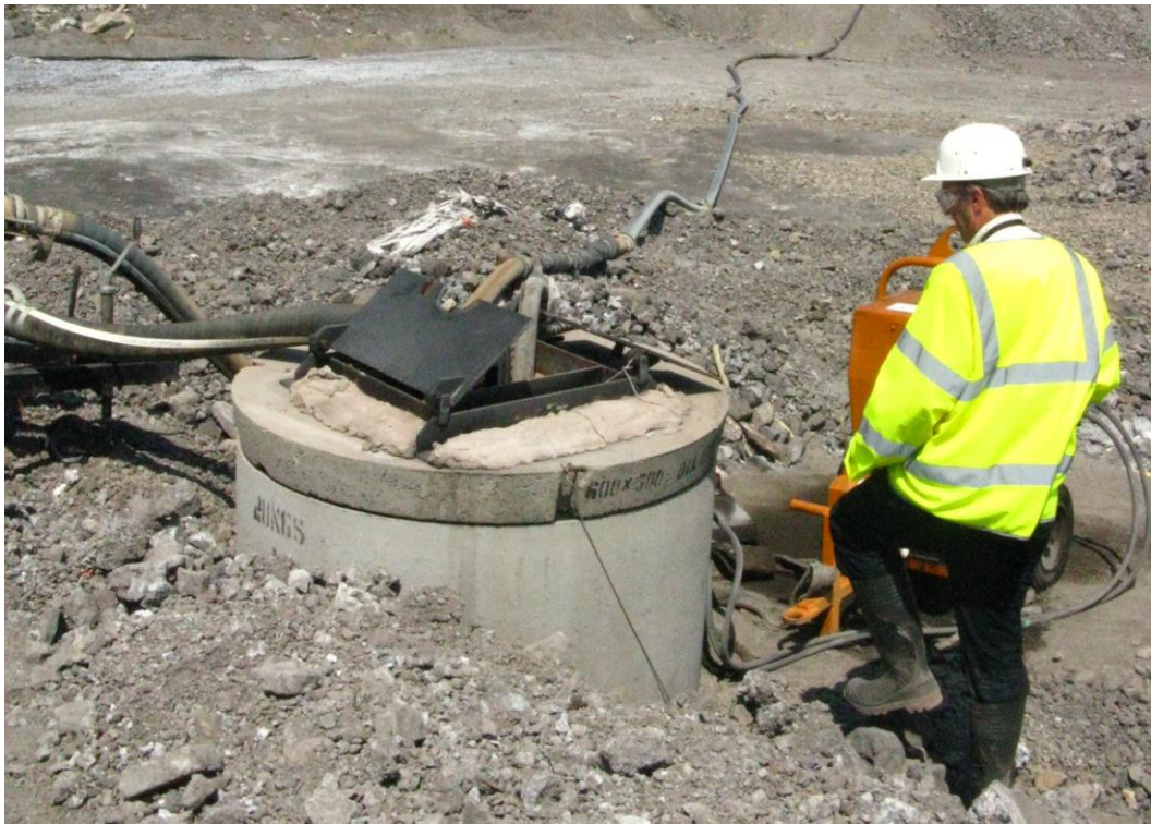
Figure 5.15 – Leachate well at Yarborough Landfill, Tata Steel, Scunthorpe
