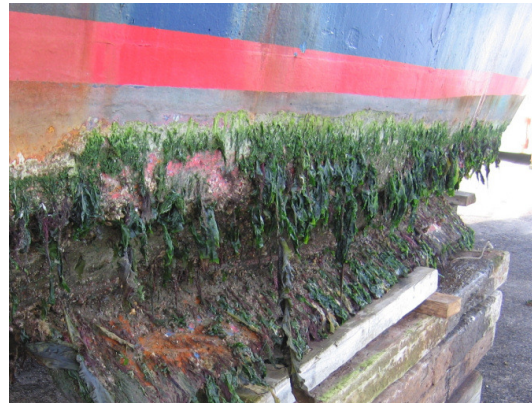
Figure 3.9: Severe weed & shell fouling
