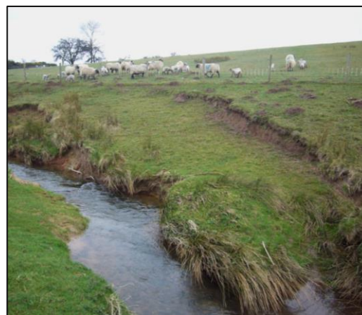
Plate 5.9: Bank slumping/mass movement at the base of Strutforth Hill, Sykeside Farm (April, 2010).
