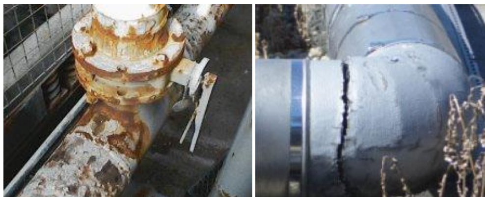
Figure 2.2: (Left) Pipe with visible corrosion, (right) pipe with damaged insulation [11].
