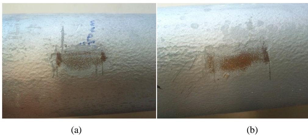
Figure 6.13: A visible sign of corrosion under the (a) top and (b) bottom tags on the un-contaminated pipe.
