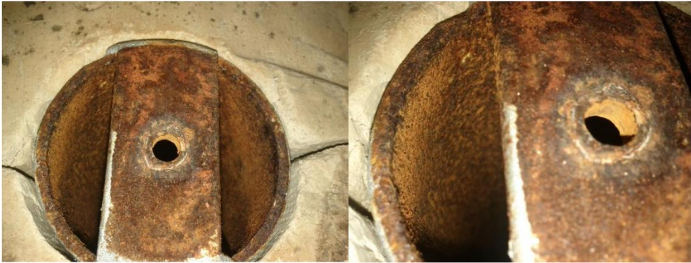
Figure 6.10: Image of the top and internal surface of the one of the pipes showing significant corrosion development after 25 days.
