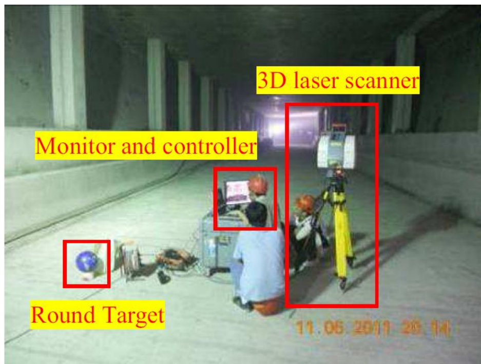
Figure 2-13: 3D laser scanning for tunnel structure monitoring (Xiongyao and Chenchao, 2012).
