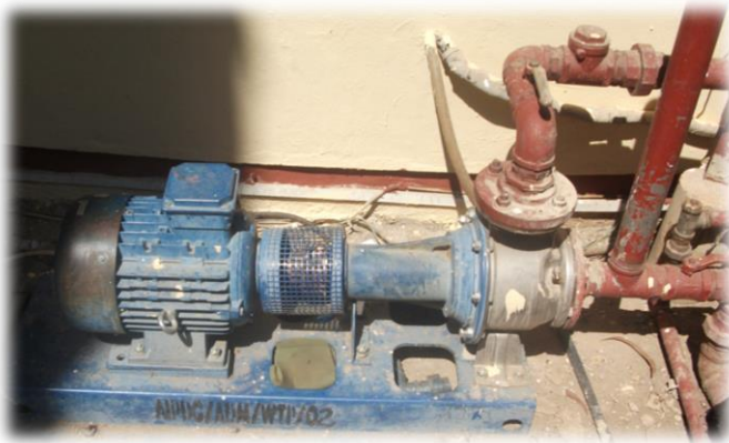
Figure 5-8 Water pump to back-up central water supply which also is scarce
