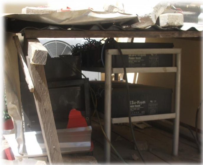
Figure 5-9 Makeshift battery storage for ICT showing poor positioning in the heat of the mechanical cooling system's exhaust and weather elements
