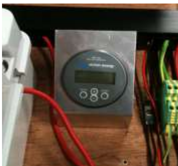
Fig. 4.14 (c) Battery monitor
