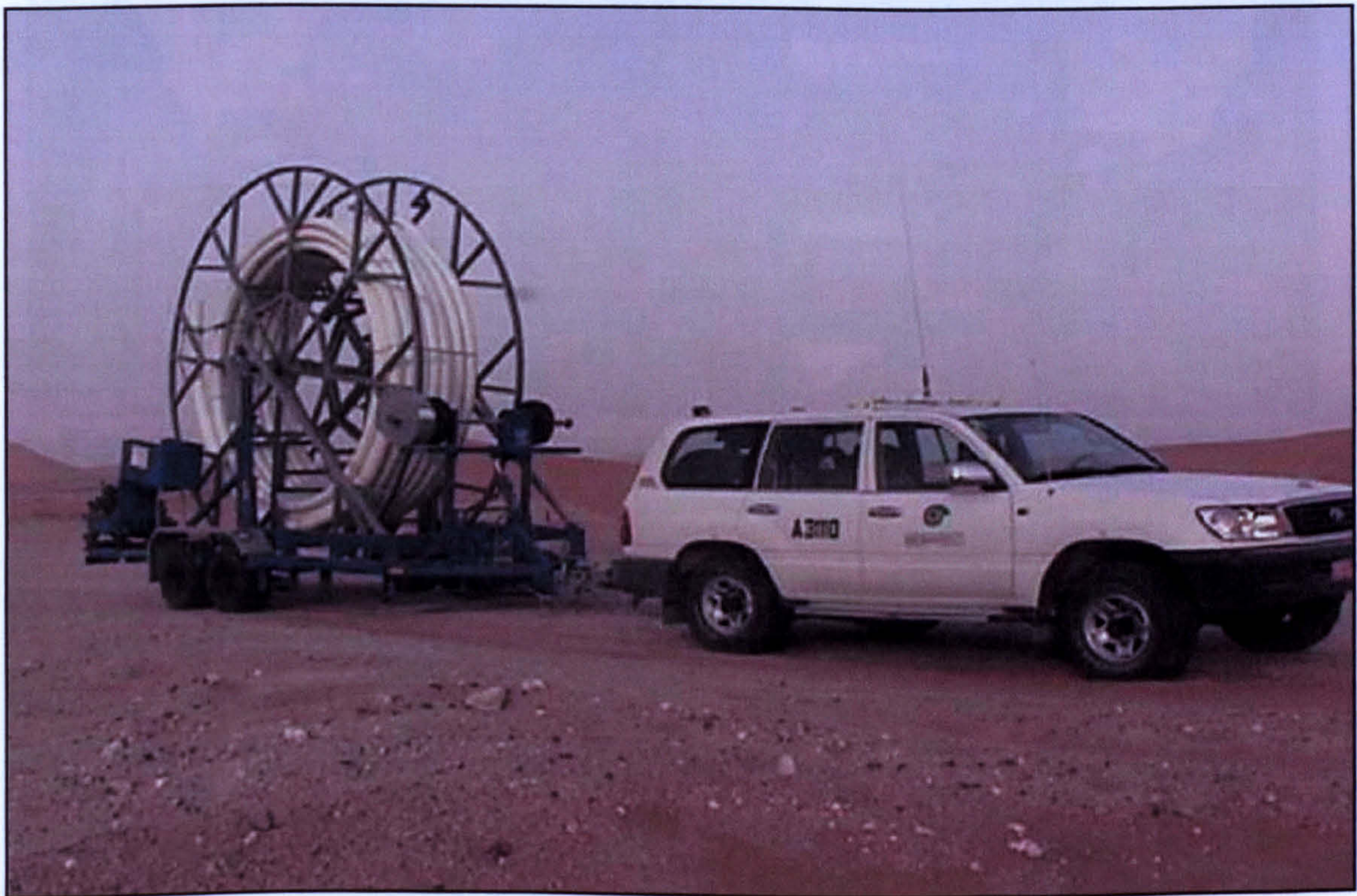
Figure 2.5 600m long 4" ID coiled RTP installed on winch towed by A 4WD for one of PDO's Oman applications (courtesy of PDO)
