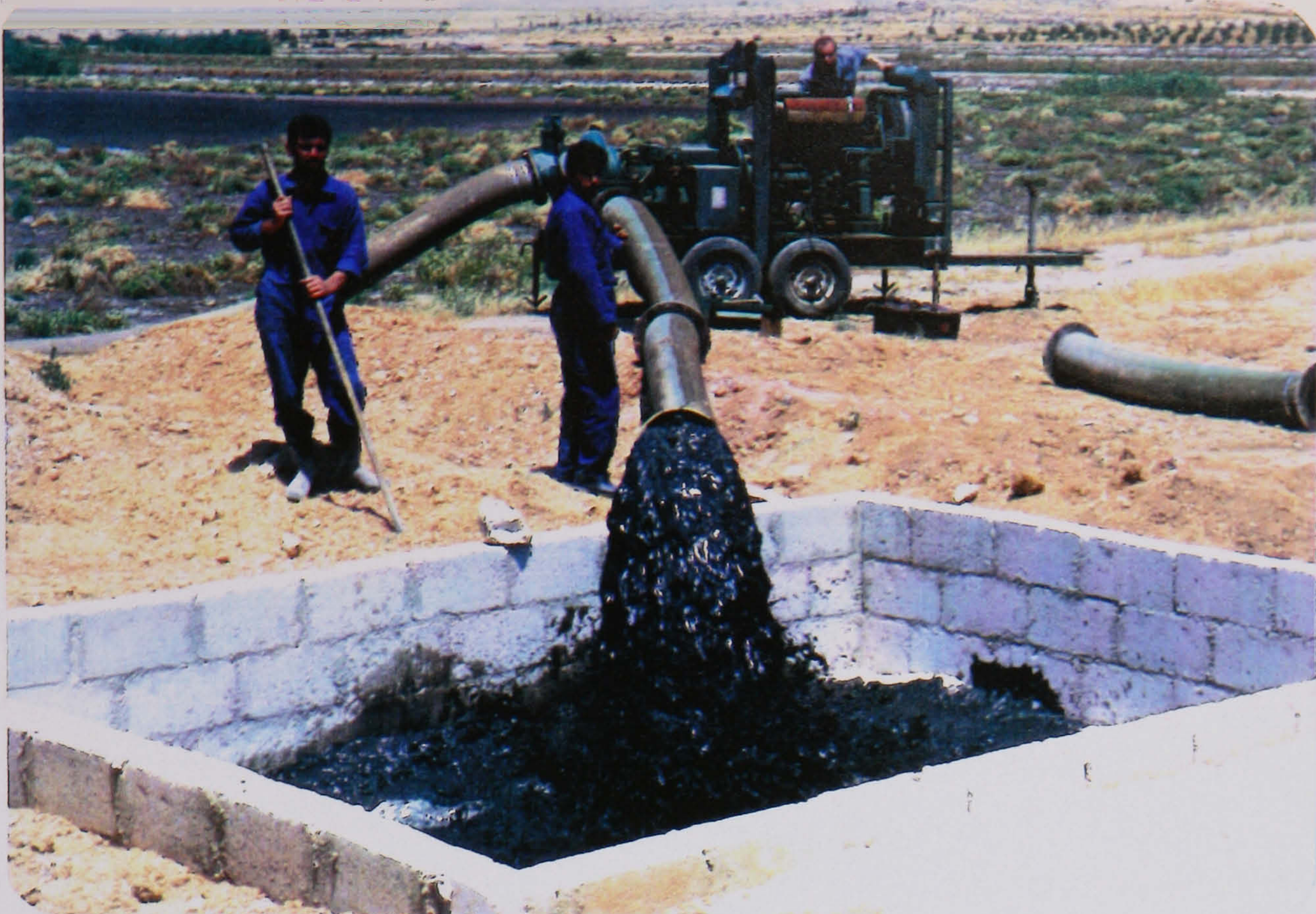
FIG. 11.23. View showing the system for pumping the anaerobic pond sludge to the ASWSP drying bed
