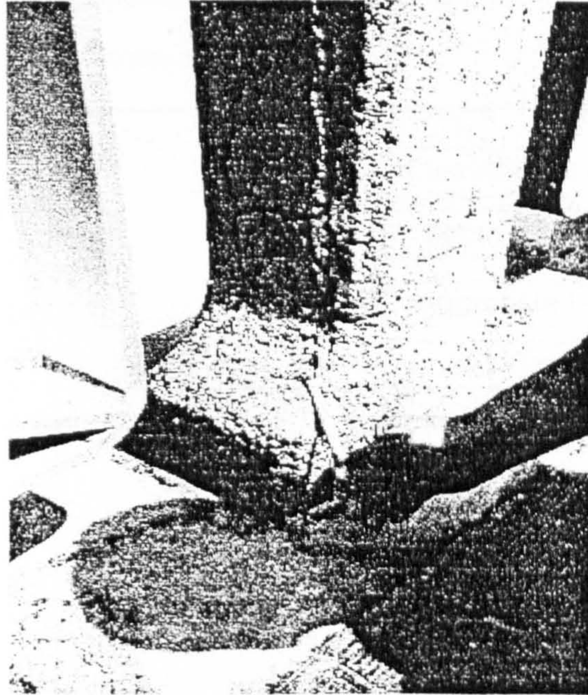
Figure 2.6 - Cracking owing to severe corrosion of reinforcement in concrete column.
