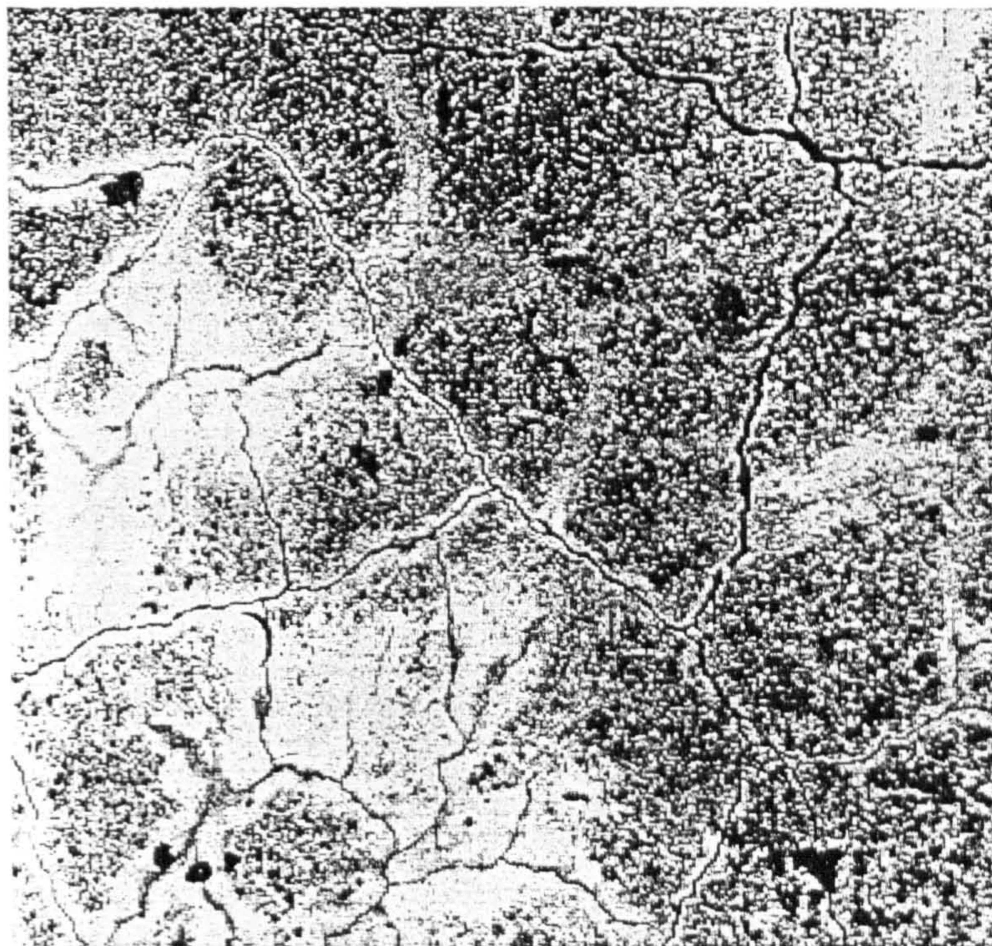
Figure 2.7 - Map cracking typical of Alkali-Silica Reaction (ASR).
