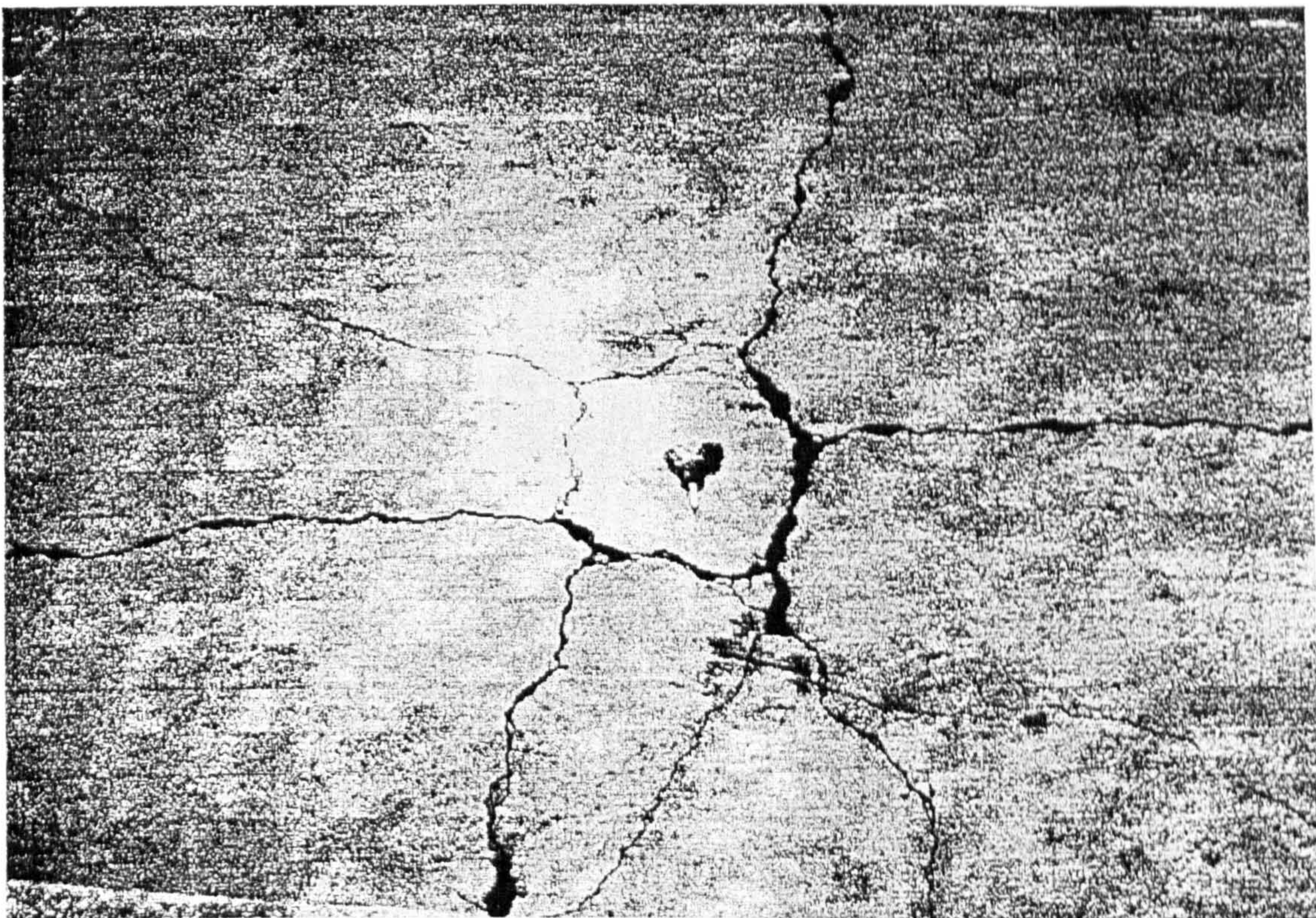
Figure 10.42 – Pattern of cracking around a local hard spot (Knapton, 2001).
