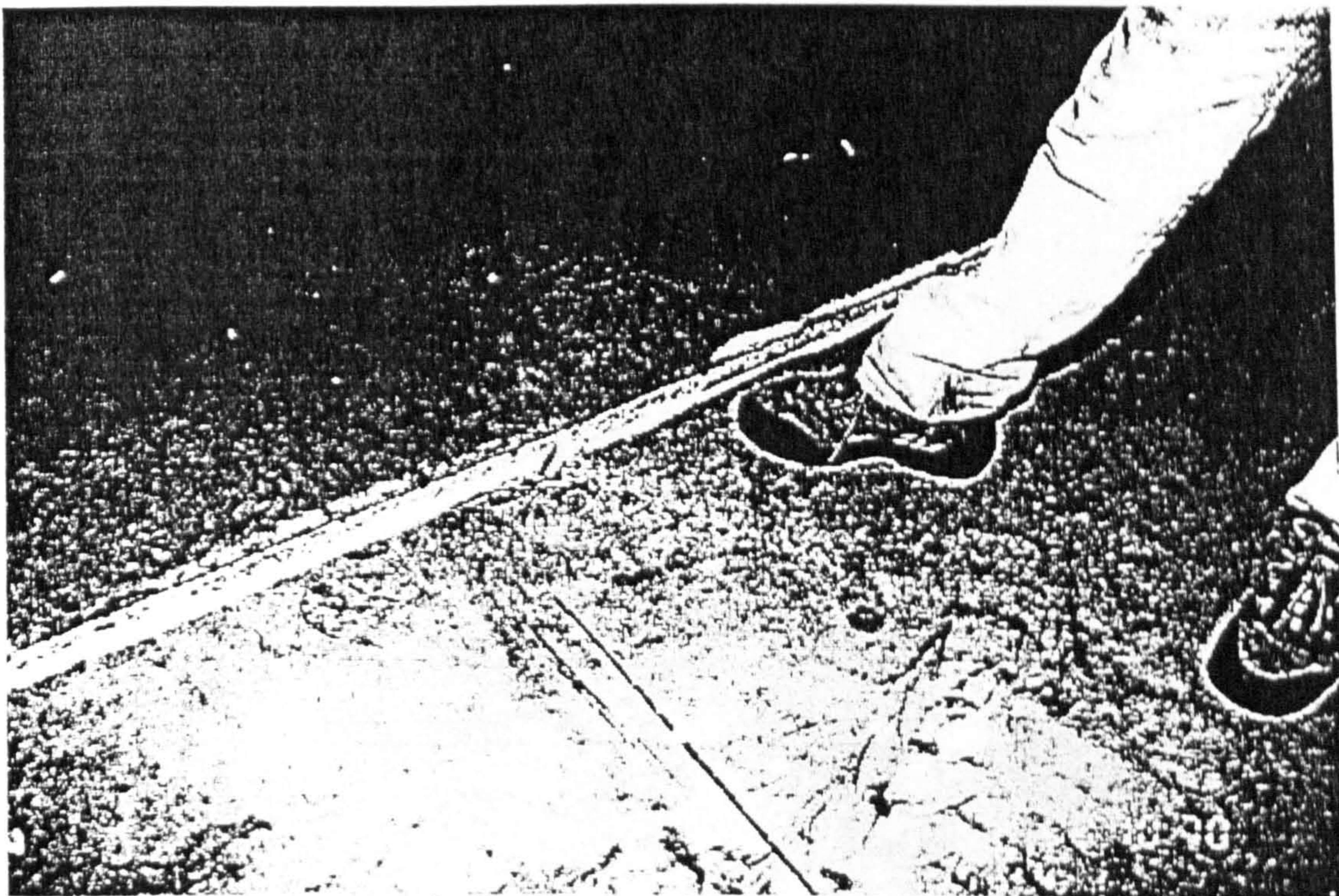
Figure 10.39 – Difference in level at cut joint and spalling at crack (Knapton, 2001).
