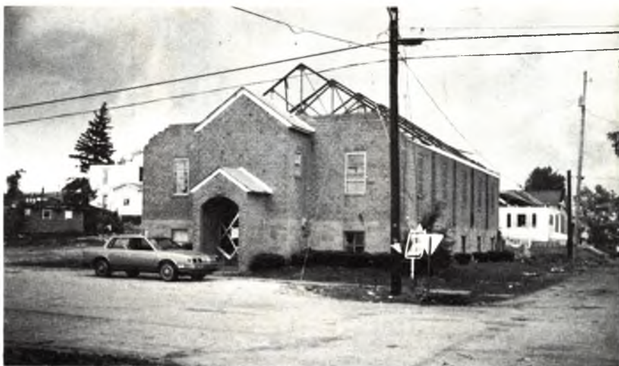
The Petersburg, Ind., Church of the Nazarene suffered extensive damage from a tornado June 2. The building, valued at $150,000, has been declared a total loss.
