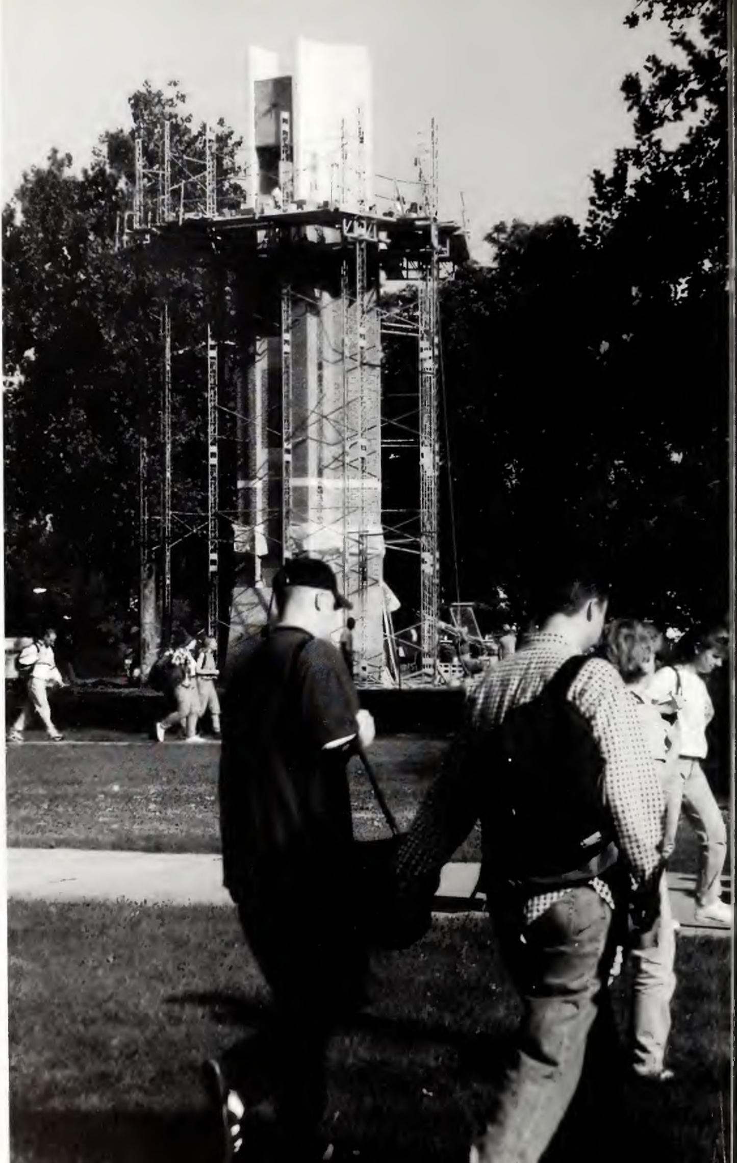
Crossing the Esplanade, students walk around the construction area surrounding the Milby Clock Tower. The tower was renovated this year; brick was put up around the original tower, and a roof and weather vane were added.
