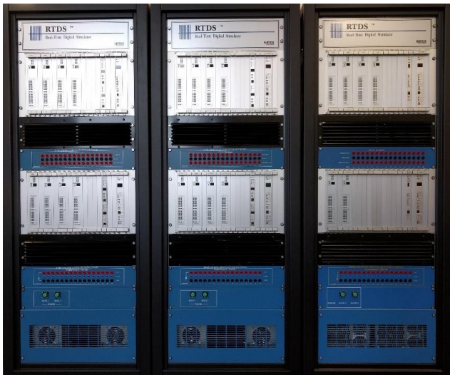
Figure 1 RTDS Hardware (cubicles)
